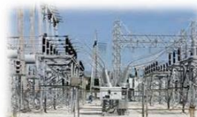
Large Scale Substation
